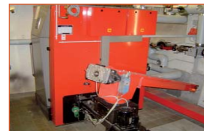
Medium-scale pellet heating system (picture: WIP)
